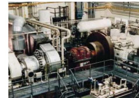
4HG compressor for gas storage driven by GE PGT5 gas turbine.
