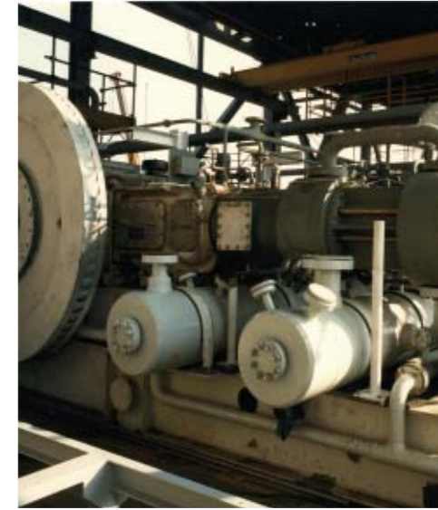
Re-injection compressor - model 6HE/2 at 415 bar.
