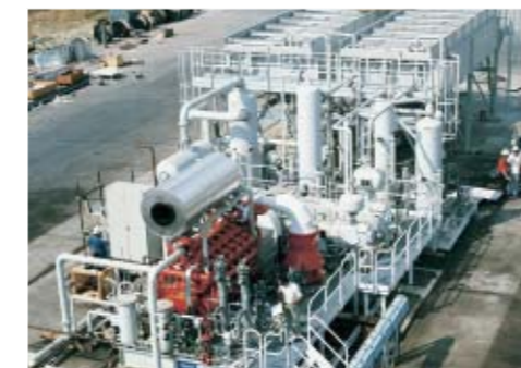
Three-stage gas engine driven reciprocating compressor for gas lift service.
