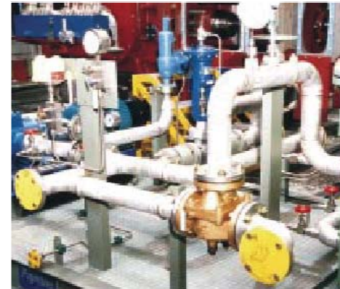
Lube oil console.
