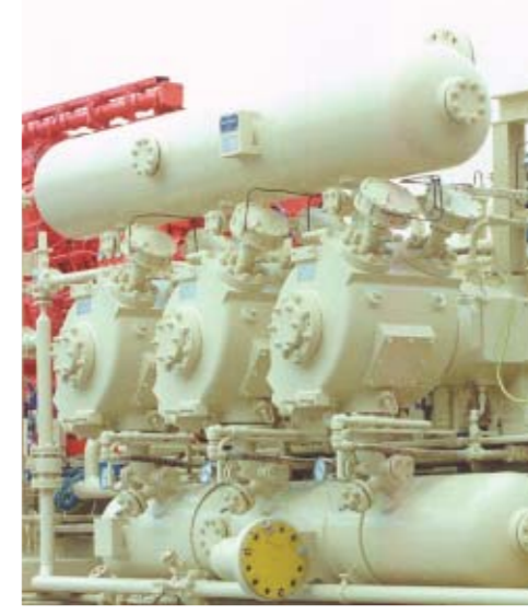
Gas gathering-engine driven high speed compressor - model 6HM/1 at 71 bar.
