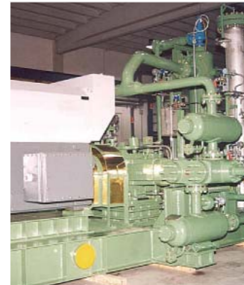
Fuel gas boosting compressor - model B452 at 50 bar.
