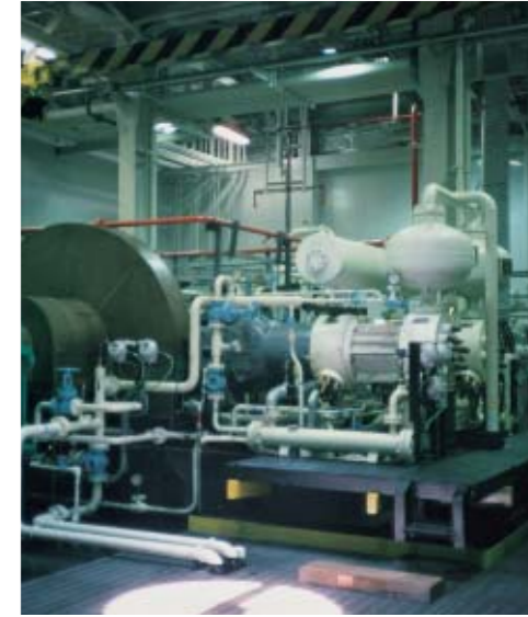
Offshore gas turbine driven compressor - model 4HE/2 at 280 bar.
