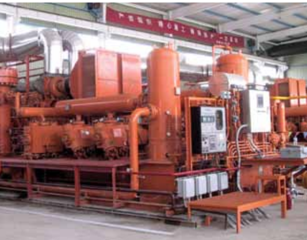
Six-throw HOS compressor installed in China.
