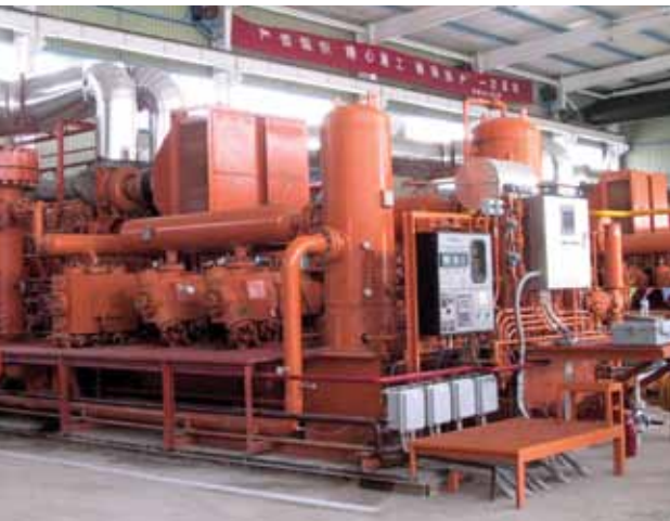
Six-throw HOS compressor installed in China.
